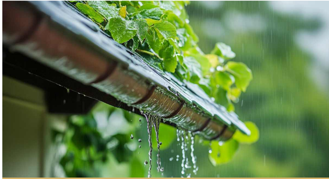
RAINWATER HARVESTING SYSTEMS THROUGHOUT
